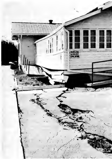
Photo 45. Damage to old wood frame structures of Olive View Hospital.
